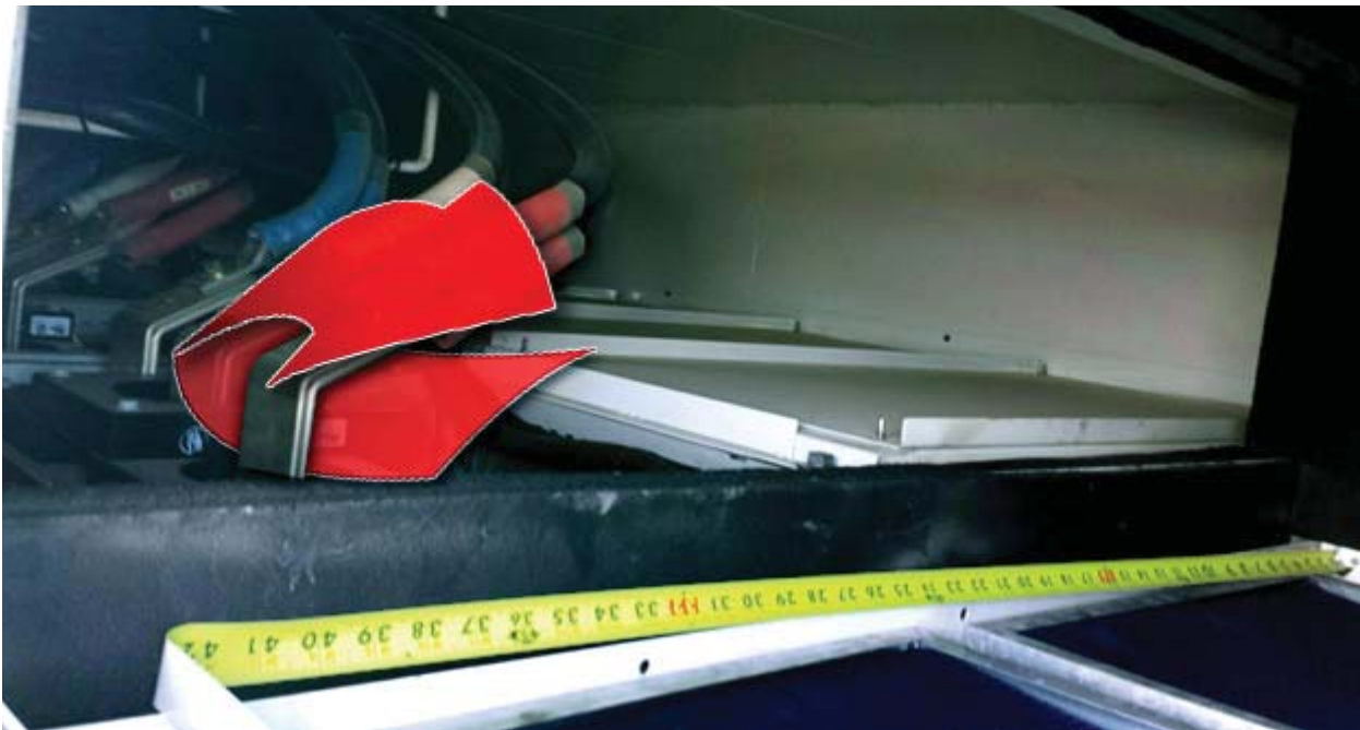
Figure 1: Have qualified personnel use insulated blanket (Canrig P/N: E16601) to completely cover the exposed conductor indicated and prevent against accidental contact.
